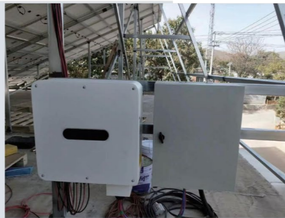
Residential PV Project in China
