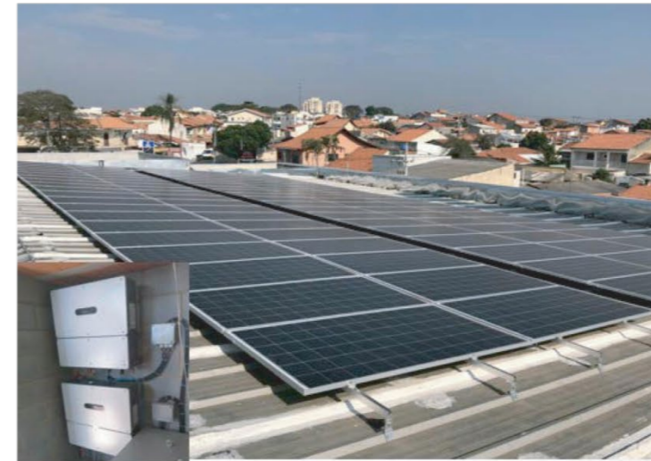
Brazil 500kW Rooftop Project
