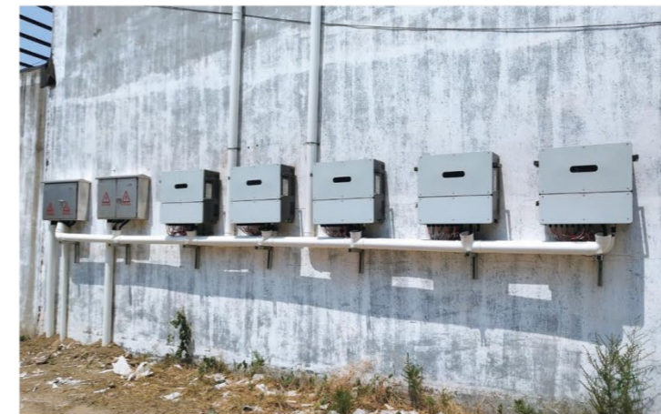
Rooftop PV Project in Shandong
