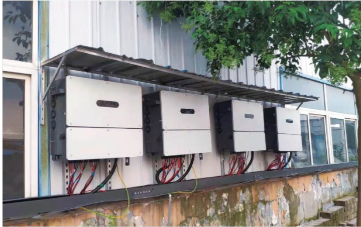
Roof-top PV Project in Dingyuan, Chuzhou, Anhui Province
