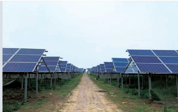
Solar Renewable Project in Anqiu
