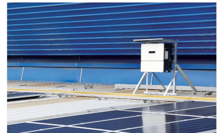
12MW Dalian Roof-top PV Project in China
