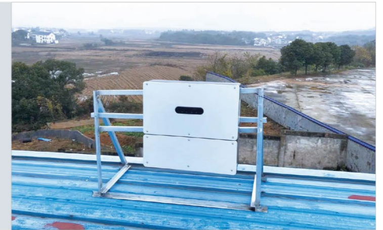
Roof-top PV Project in Hunan China
